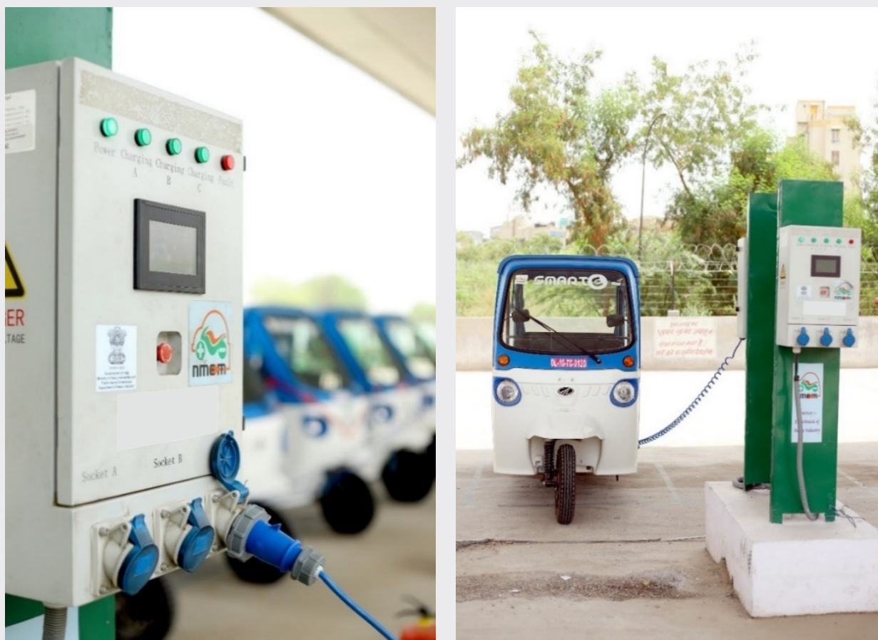
FIGURE 16 | Charging infrastructure for e-autos in Delhi
